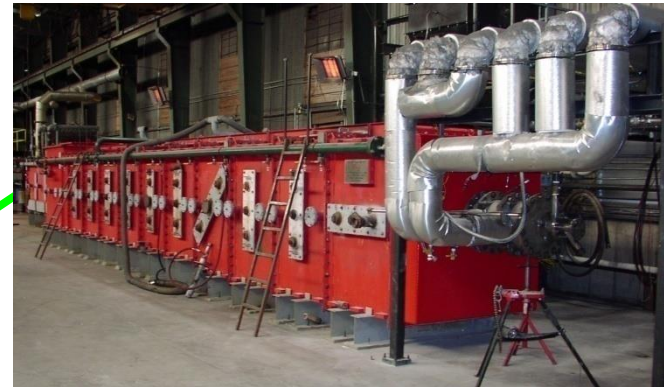
1.5 MW pulverized coal furnace (L1500)
